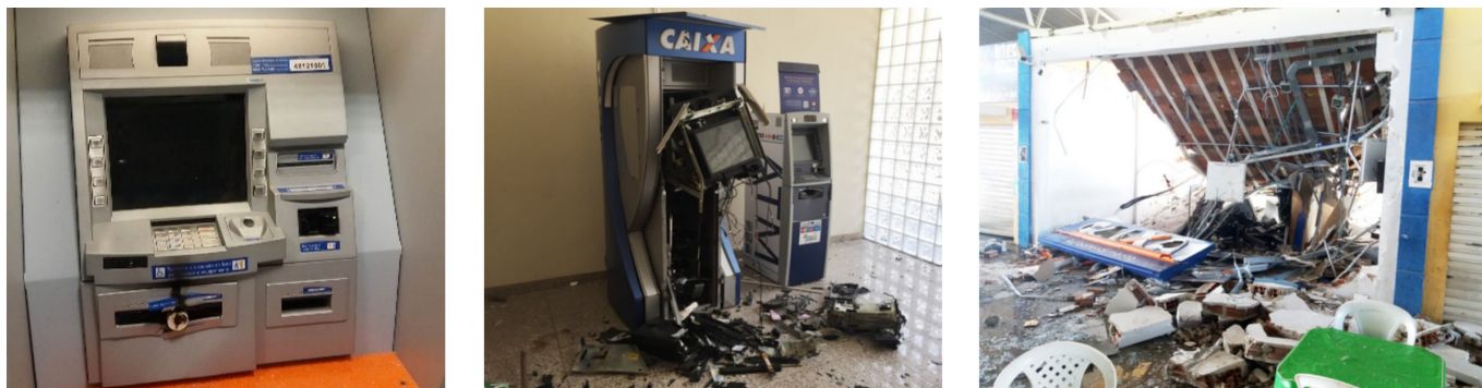
Figure 1. Unsuccessful ATM explosion attempt (left), 4 effective ATM explosion with relative level of destruction (center) 5 and ATM explosion with high level of destruction of a bank branch with damage including its building structure (right). 6
